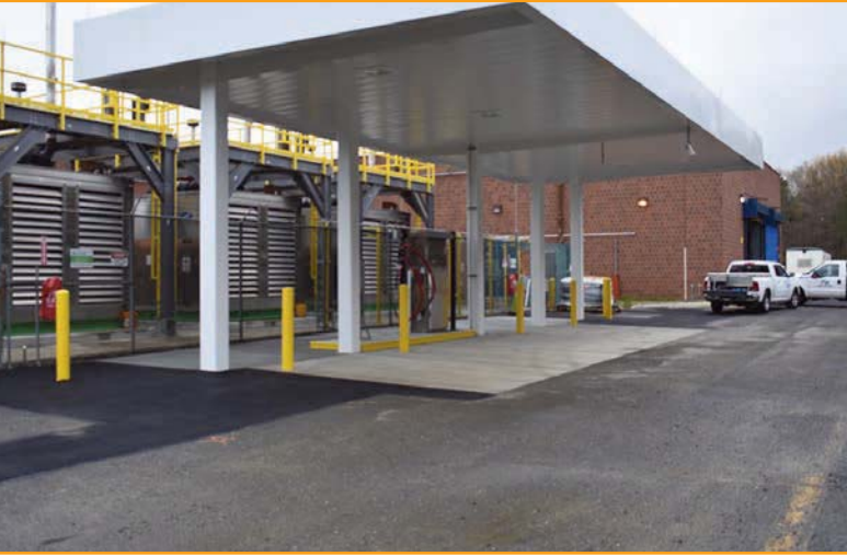
West Bay installed concrete foundations for three new compressors in the background and the new fueling canopy at the NJ Transit Howell Bus Maintenance Garage.
