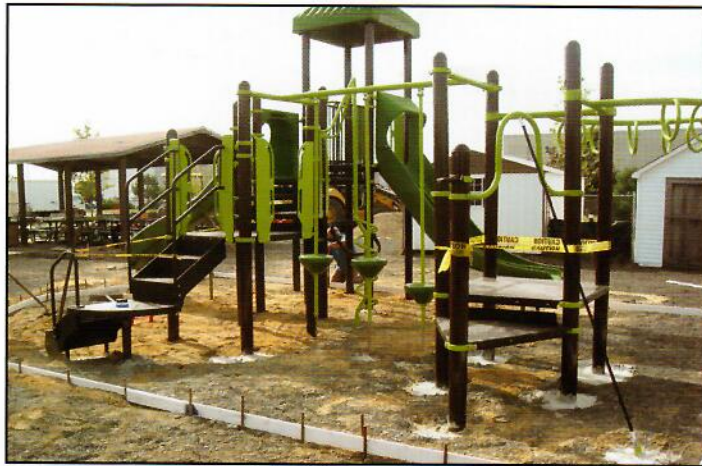
A playground is constructed for the U.S. Air Force at the Joint Base McGuire-Dix-Lakehurst.
