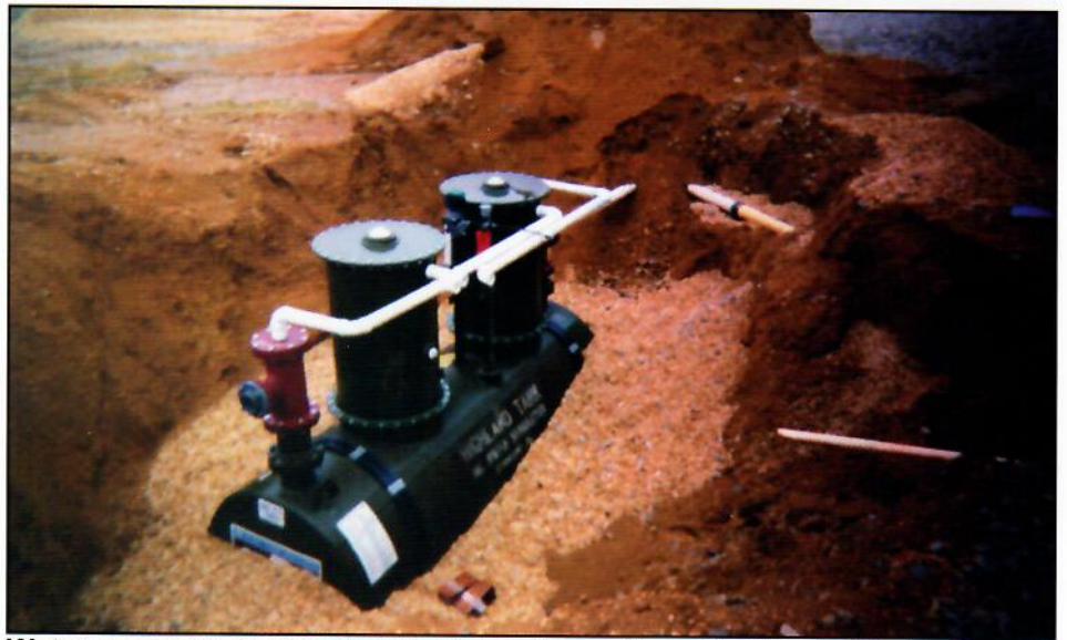
Water separator installed at the NJ National Guard facility in Vineland.
